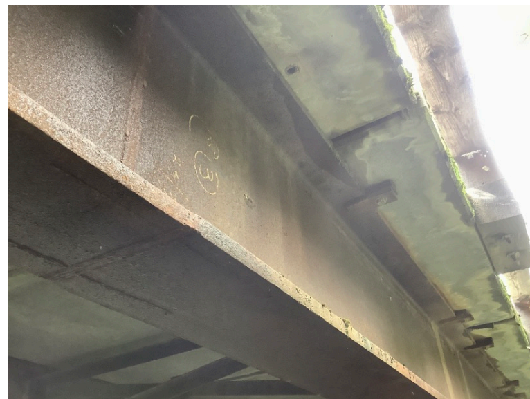
Deck - missing deck bolt and plate
